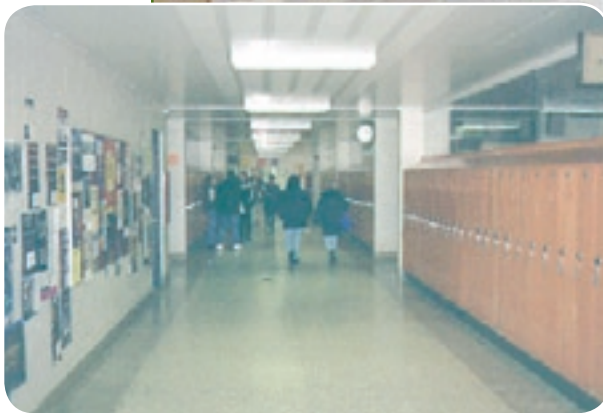
Existing, low ceiling corridors. The challenge was to incorporate mechanical and electrical upgrades.
