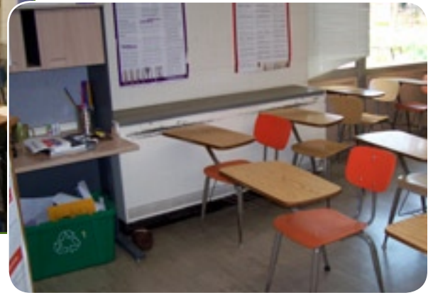
Old horizontal unit ventilators
